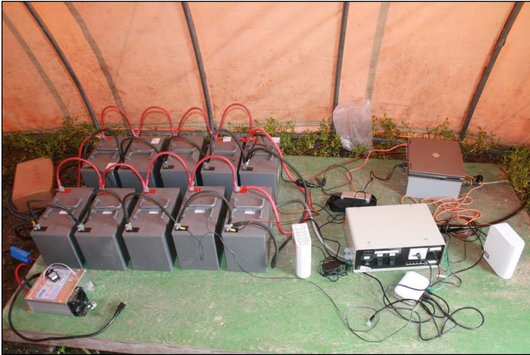
Photo 7. Control box, NAS, and power source housed in the WeatherPort tent, 2011.
